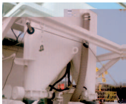
Cement and water weighing system
