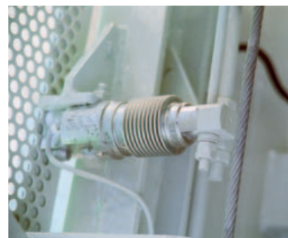
Electrical measurement device
